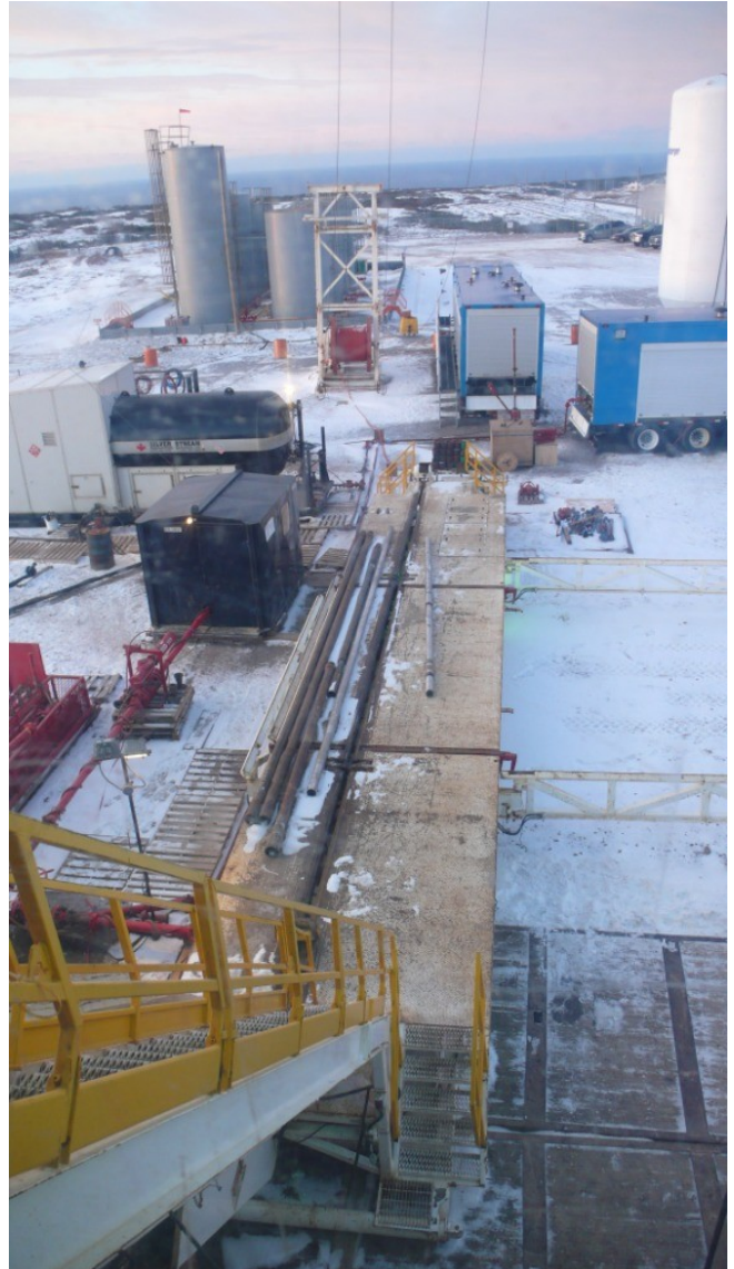
4 – GRT Tool on the catwalk
